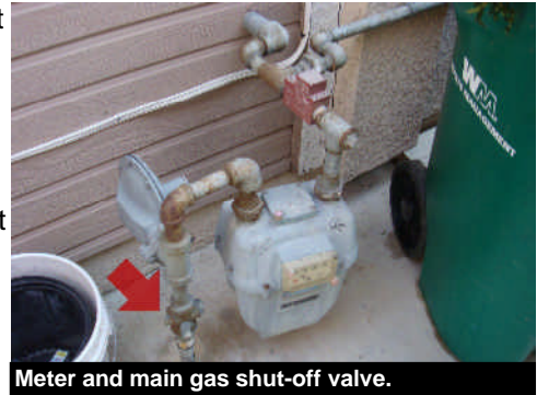
Meter and main gas shut-off valve.
