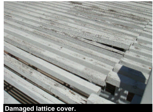
Damaged lattice cover.
