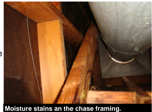
Moisture stains on the chase framing.
