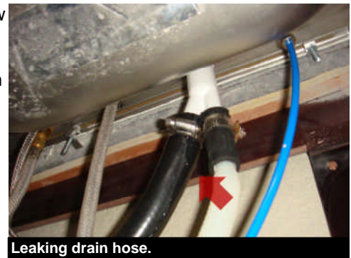
Leaking drain hose.
