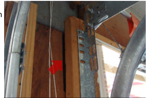
No backing behind the support block.
