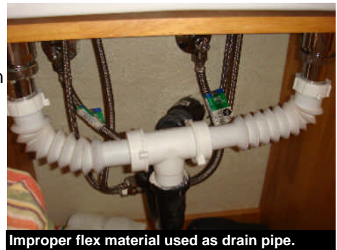
Improper flex material used as drain pipe.
