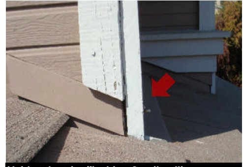
Void at the trim /flashing & nail pulling.
