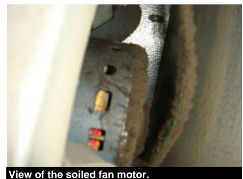
View of the soiled fan motor.
