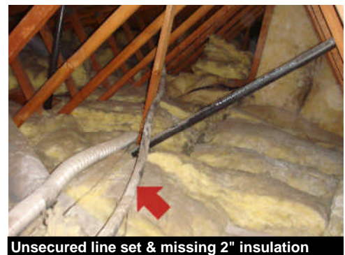
Unsecured line set & missing 2" insulation
