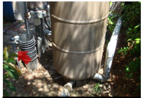
Valve may be spa fill valve. Not tested.
