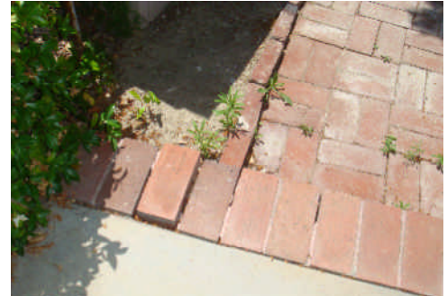
Loose bricks & missing mortar at spa.
