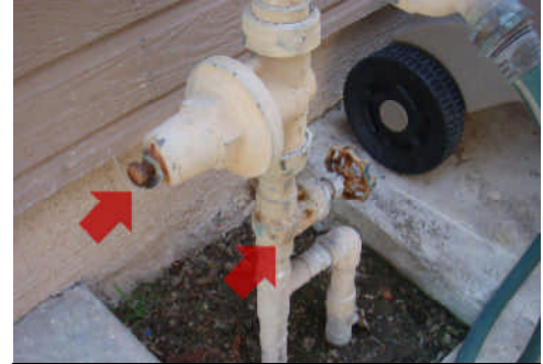
Pressure regulator and rusty valve.
