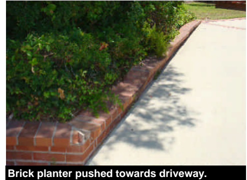
Brick planter pushed towards driveway.
