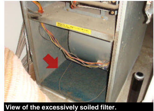
View of the excessively soiled filter.
